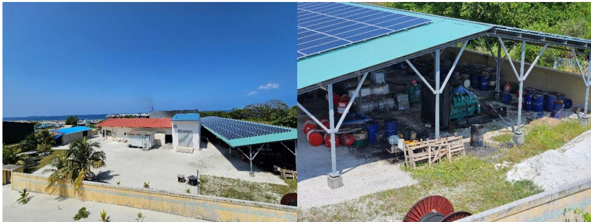
Figure 4: Used oil containers stored in Manadhoo Fenaka Powerhouse
